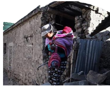
Fig.32. Collapse in corners of a building (a) Plastic deformations in the numerical models (b) Andina Peruvian news agency [1]
